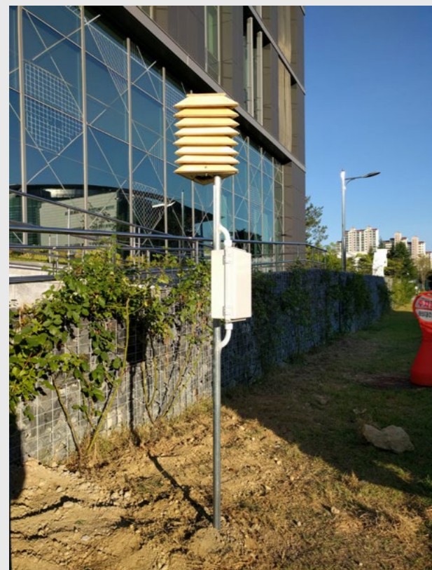
▲ POSTECH Weather Station's Ground Monitoring Unit (Jul 2017) Bodenstation der POSTECH-Wetterstation (Juli 2017)
